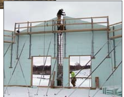
Polystyrene forms constructed and braced. Inset shows the reinforced interior of the walls prior to filling with concrete.
